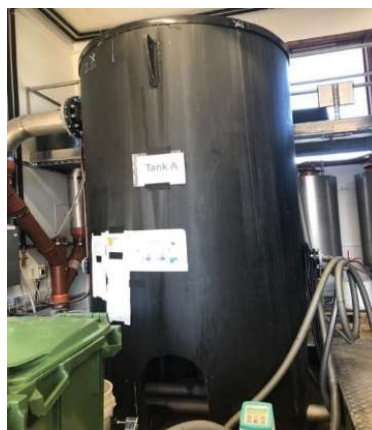
Figure 10 Wastewater storage tank in the Wastewater laboratory at Norwegian University of Science and Technology
