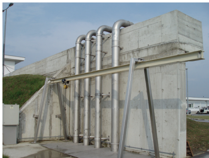
Slika 1. Crpna stanica u pogonu za obradu otpadne vode grada Vinkovaca Fig. 1. Pumping station in wastewater treatment plant of the Vinkovci town
